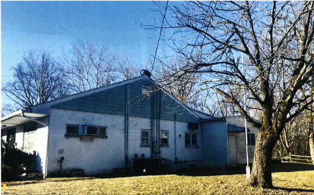
2 - Mildew and peeling paint on the northern facade
