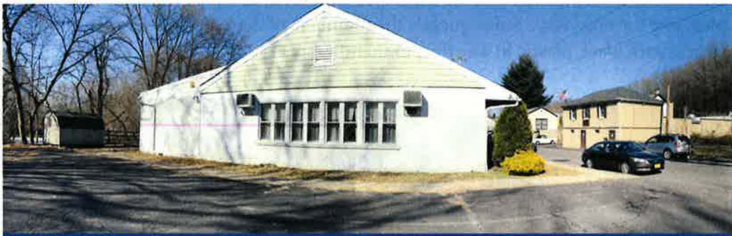
3 - Exterior damage on the southern facade
