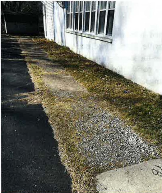
5 - Deteriorated concrete pathway on south side of the building
